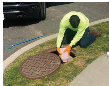
A TOSA employee adds dye to the sewer line adjacent to Deal Lake to test for leaks in the infrastructure
